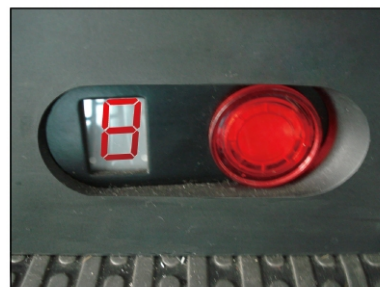
Fault Display for S and F Type
